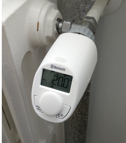
Fig. 1: EQ3 Eqliva valve on a radiator
