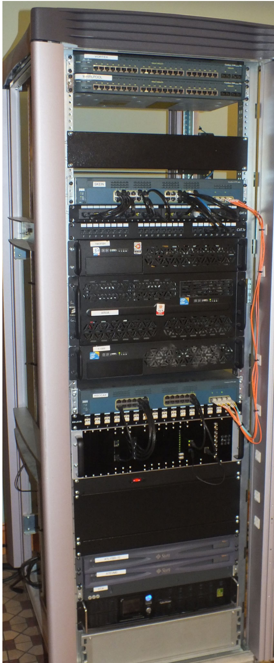
Figure 4.6: FPGA cluster on rack
