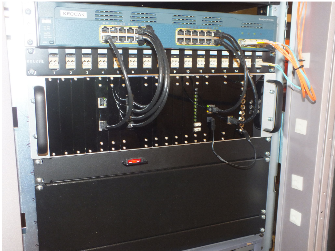
Figure 4.5: FPGA cluster on rack
