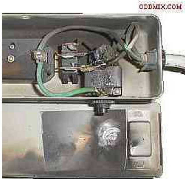
Picture 1. Open power strip
