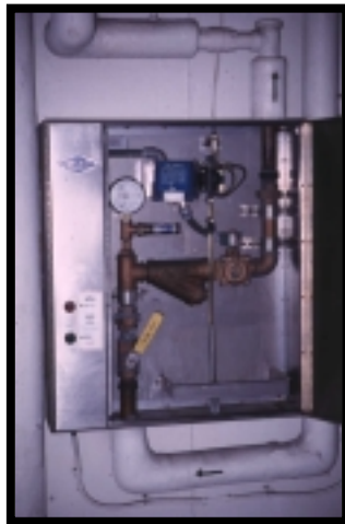
Fig. 2-10. Valve junction panel.
