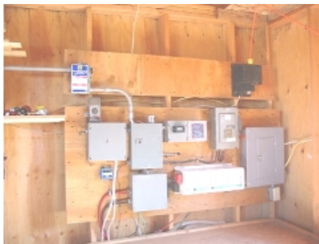
The complete control system
