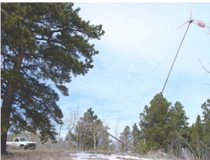
A 40-foot tilt-up tower being raised via pickup truck and gin pole. Colorado, USA
