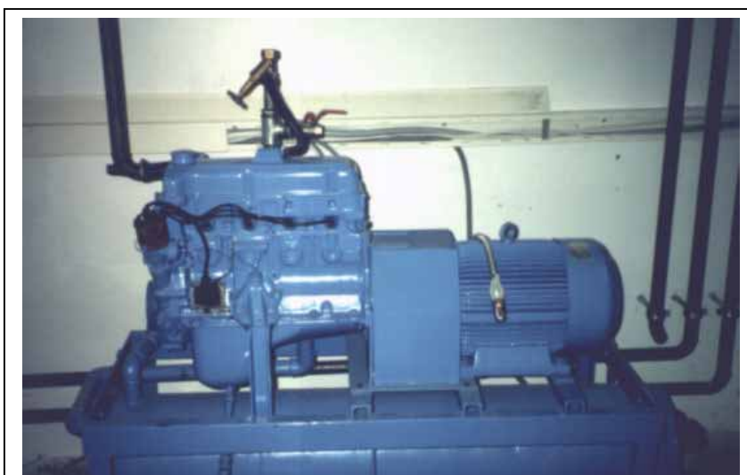
Figure 47: Co-generation unit (electricity and heat utilisation)
