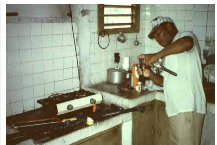
Figure 26: Final touches on a piping system with PVC pipes Photo: Krämer (TBW)
