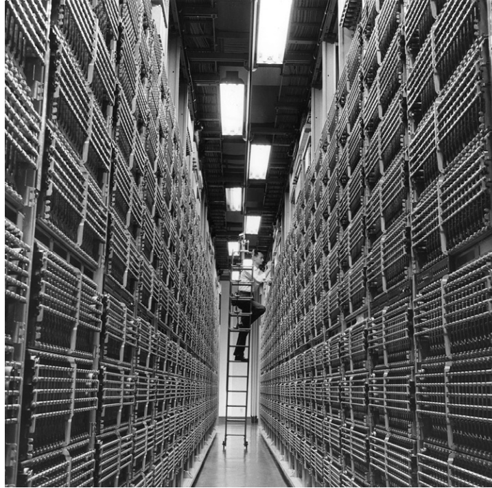
A portion of the magnificent 4A toll crossbar switch, 1957. The brains of the long-distance network, the 4A would enable truly automated long-distance telephone calls that customers could dial themselves. Photo courtesy AT&T Archives and History Center
